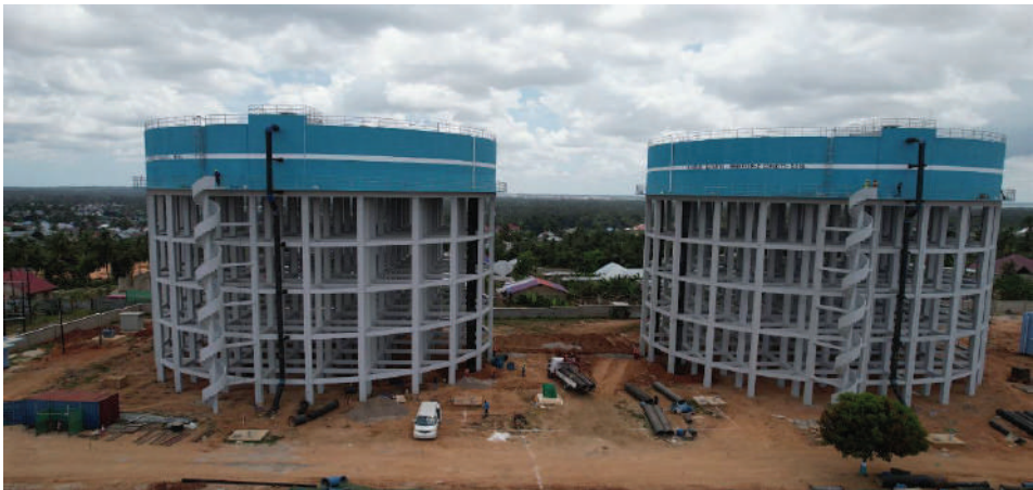
Picture 20: New Water Tanks Constructed to Boost Water Supply in Urban, West Region
